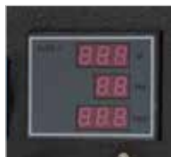
Display (voltage, frequency and hour meter)
