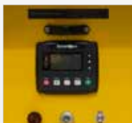
Multifunction control panel
