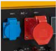
Single-phase - 230 V AC 50 Hz - Three-phase - 480 V AC 50 Hz
