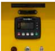
Multifunction control panel
