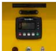
Multifunction control panel
